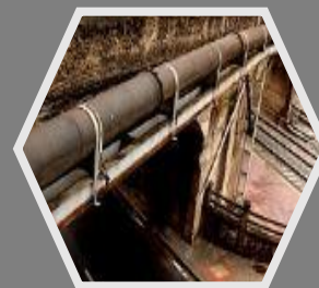
OVER 20,000 MILES OF PIPES
