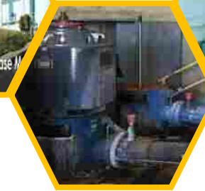
883 WATER PUMP STATIONS 714 WASTEWATER PUMP STATIONS
