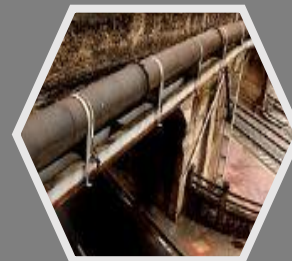
OVER 20,000 MILES OF PIPES
